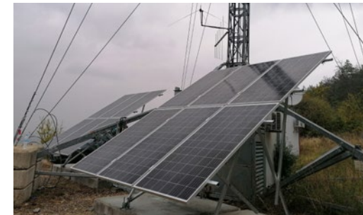
6: Vivacom, Intiman base station
